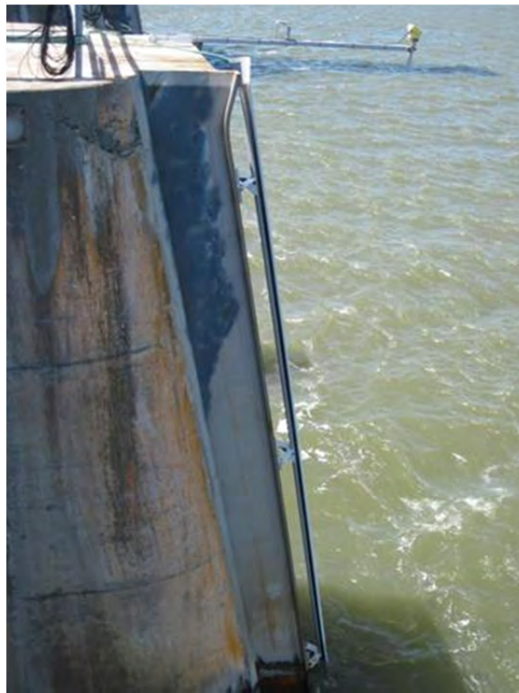
Figure 2.8. Trolley Pipe Mounted on a Main Pier of The Dalles Dam Powerhouse
